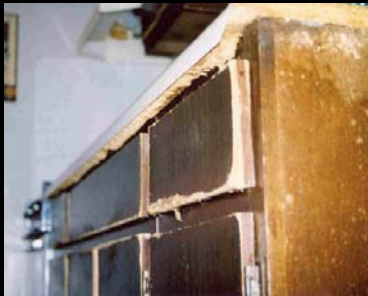
Typical damaged wood cabinets.
